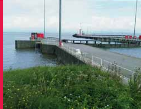
Crack Repair and Inner Dock Wall and long term Protection from water ingress, at Bristol Port, UK
