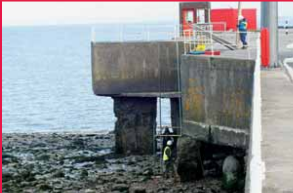
Repair and protection of support columns from further coastal erosion of the West Stub Pier , Bristol Port, UK
